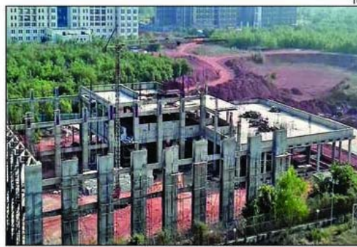
Besides grand classrooms, the IIT-BBS administrators have also expedited construction of three new school buildings
